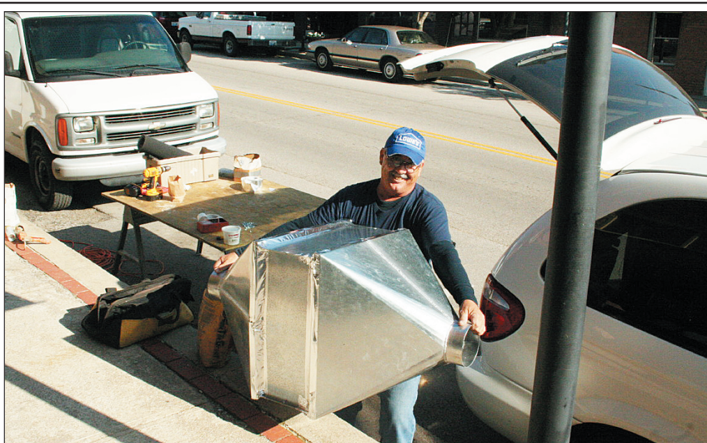
Danny Elam, who was working for DocAir, carries a portion of a new heating and cooling vent into the Jones Building on Main Street in Mt. Vernon on Monday. Work is underway on that building and the building which houses Ashlee's House because of gas fumes on those buildings. Contractors have also been installing exhaust systems behind some buildings on Main Street in order to pull more fresh air into the buildings.
