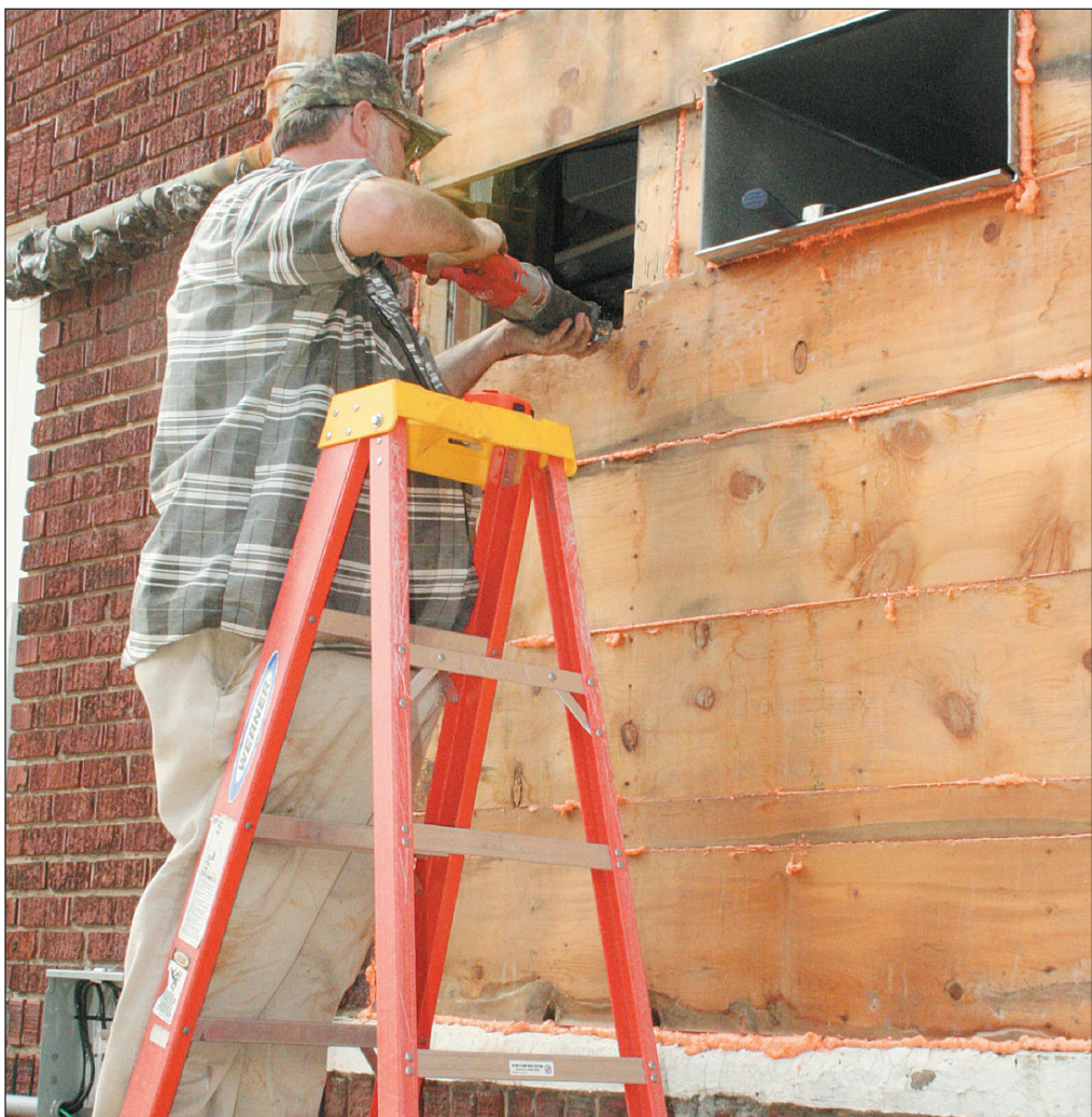
Gary "Hoss" Hurley, an employee with Winstead's Heating and Air, worked to replace heating and cooling vents in Dr. Parsons' office, as part of the work on the dentist office to try and rid the building of gasoline vapors. The office was closed for three days because of the work, but has been re-opened.
