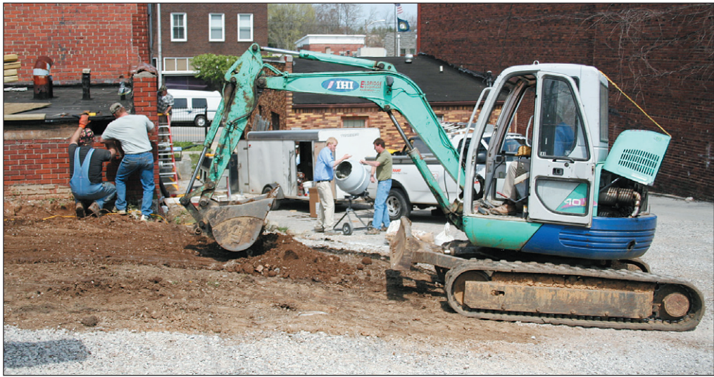
Employees of Chase Environmental and DocAir were in Mt. Vernon last week at the request of the State and Federal EPA working on the building of Dr. John Parsons, which is located on Main Street in Mt. Vernon. The work was being done to try and rid the building of gasoline vapors, which have been a problem since 1994.
