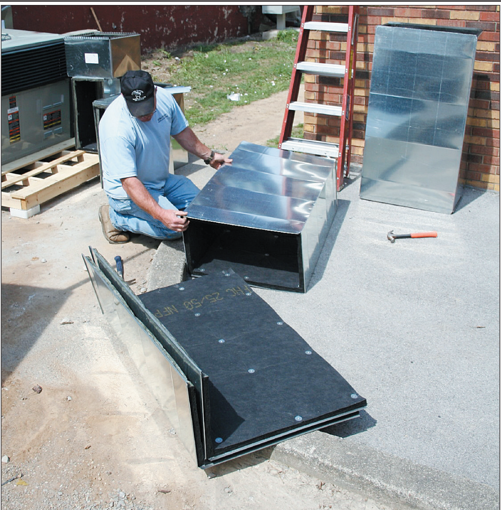
Burley Burkhart, an employee with Winstead's Heating and Air, was one of many people who worked on Dr. John Parsons' building in Mt. Vernon last week. The work on Parsons' building and the property around it cost approximately $52,000, according to officials, who said the EPA is footing the bill. (Photos by: Richard Anderkin).
