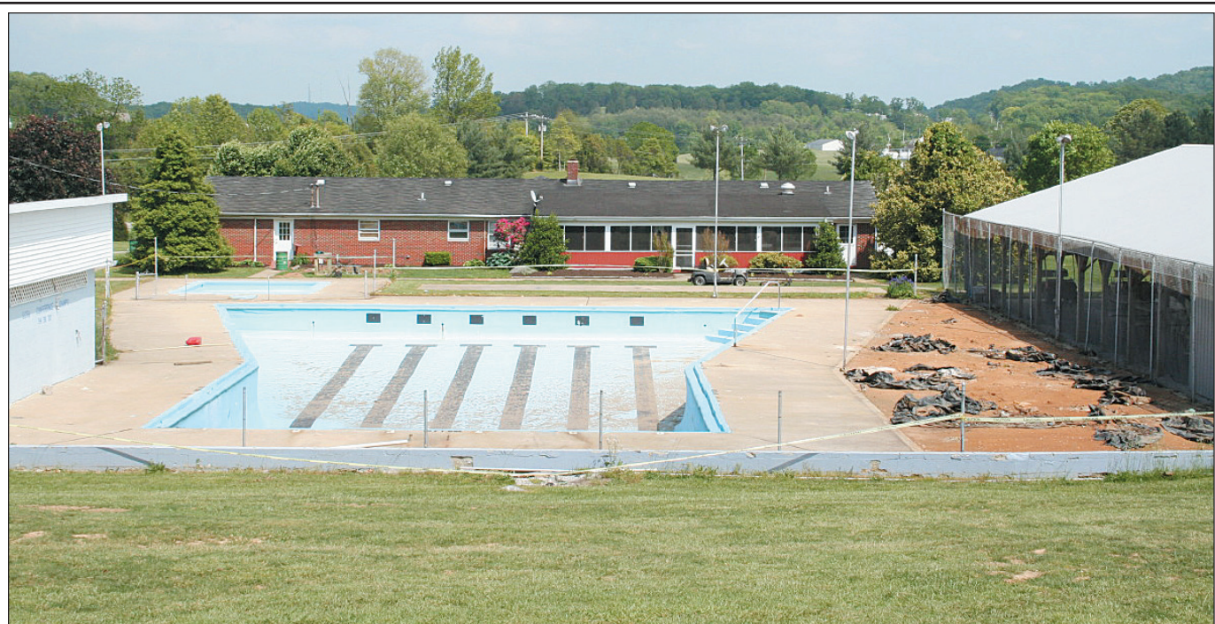
Work to repair and renovate the swimming pool at CRRC had already begun when the state stepped in and shut down the renovaton project a few weeks ago. It is not known when or if the pool will be ready to open this summer.
