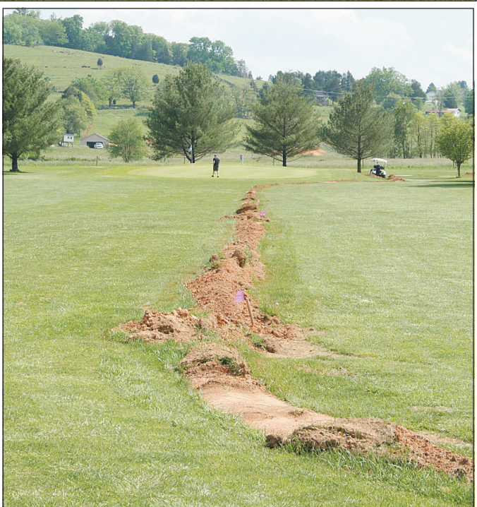
Except for smoothing down dirt in the fairways, work on a new irrigation system for the golf course at CRRC has been completed.
