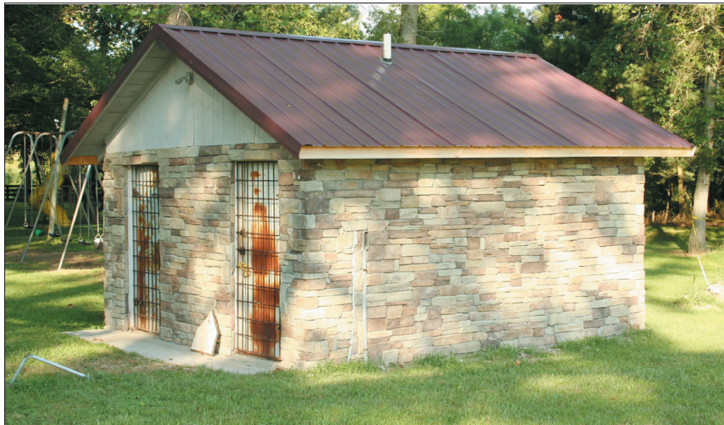
New stone has been put on the exterior of the bathrooms at Quail Community Park as part of the construction and remodeling project now underway.
