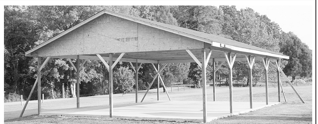
A new outdoor shelter is under construction behind the Cupps Chapel Church building. Labor for the construction was donated by Dennis Doan's crew. Offerings for the materials were received during a recent revival at the church.
