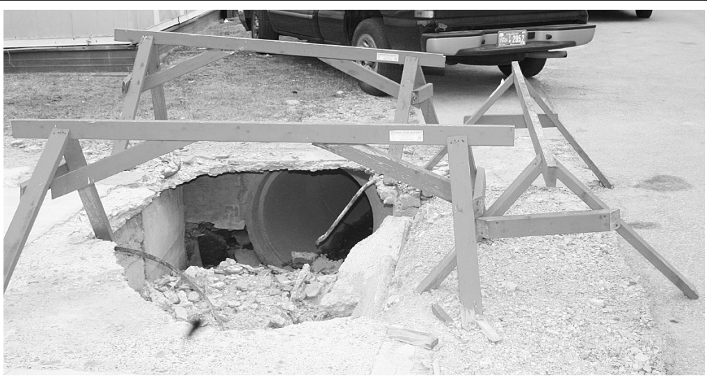
Motorists should be aware of a huge hole on Church Street in Brodhead, which has not been repaired. According to Mayor Walter Cash, a Bee Garbage truck got stuck in the hole recently, after the pavement collapsed while it was picking up a garbage dumpster. Church Street runs into Main Street, along buildings which house, Collins Respiratory Care and Marsha's Florist.
