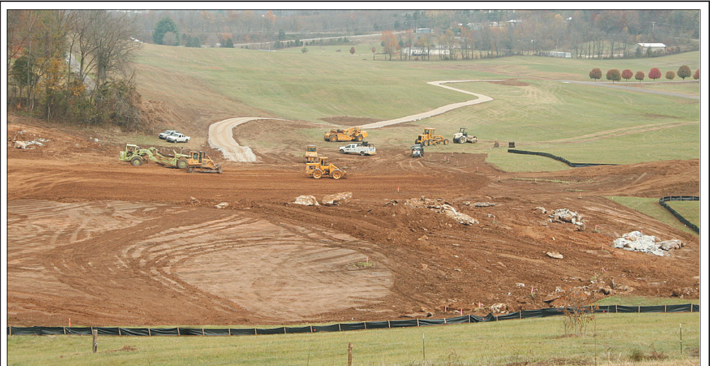
Work is well underway in Industrial Park South off old 461, on the site where a new building will be built for SourceCorp. The company is expanding its operation in the county and approximately 140 new jobs will be created. Larry Goff Construction has the bid for the site preparation and construction of a temporary road to the new facility, which is scheduled to open sometime in late spring or early summer of next year.
