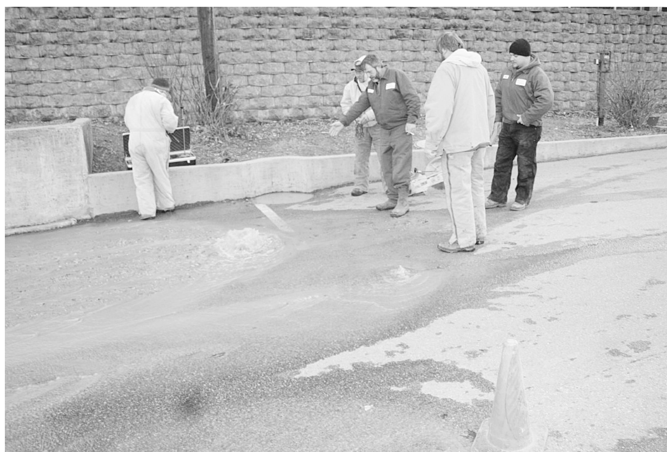
Mt. Vernon Water Department employees spent several hours on Thursday evening repairing a water main break on Main Street in Mt. Vernon. Above, City Superintendent Dennis McClure instructs workers on how to proceed in repairing the ruptured line. McClure said it was hard to determine, but that he estimated several thousand gallons of water was lost because of the hole in the bottom of the line. Thursday's break was the worst so far for the city this winter, which has fared extremely well in that department, according to McClure.
