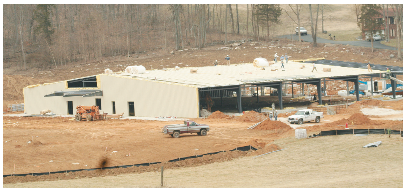
Project Manager Jim Holton told the Rockcastle Industrial Development Board of Directors on Monday, that although some construction problems have been incurred and the weather has not cooperated, the new Sourcecorp building, shown above under construction, is still close to being on scheduled for completion in June. (Photo by: Richard Anderkin)
