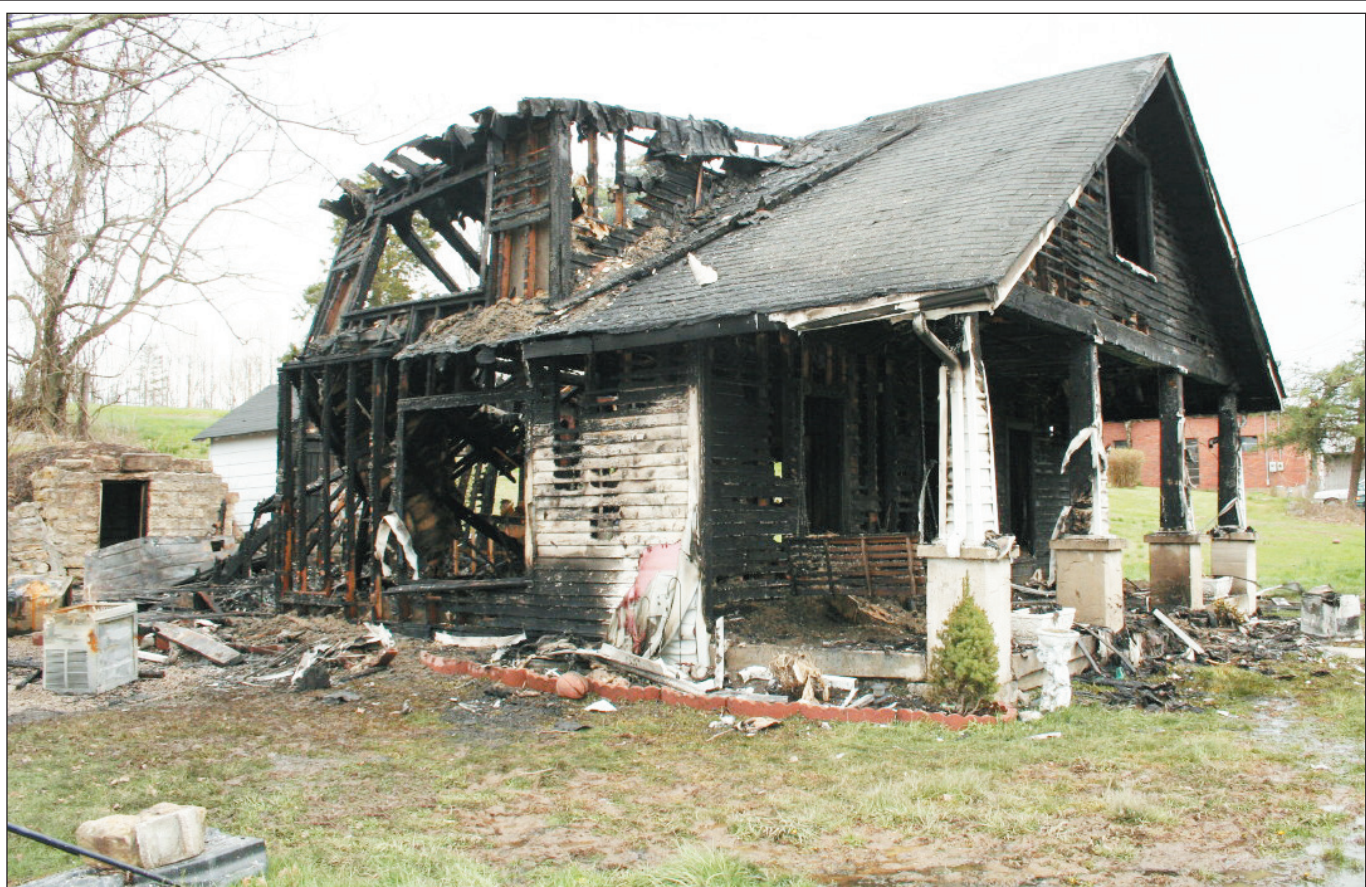
Sandy McClure and her two sons lost everything in a fire at their home in Mt. Vernon early Tuesday morning. Their home, shown above, was completely engulfed when firefighters arrived at the 3 a.m. fire.
