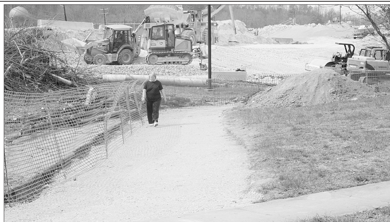
Lavada Gatliff, one of the many local residents who make a routine out of walking at the city park on Williams Street in Mt. Vernon, walked around the make-shift gravel track last week, while construction was going on behind her at the Hanson Aggregate Quarry. A Hanson official said Tuesday the $6 million renovation project, now underway at the local quarry, should be completed around the end of June. As part of the renovation and expansion project at the quarry the city of Mt. Vernon gave Hanson approximately one tenth of an acre to make it easier for CSX train cars to come and go from the quarry. In exchange for the park property, Hanson agreed to do all of the work involved in the project, which includes shortening the track and give the city 100 tons of materials from the plant each year for the next five years. Hanson officials has said they would not fight annexation into the city of limits of Mt. Vernon.
