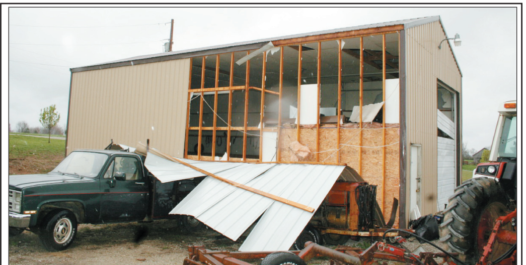
The workshop at S & S Excavating on Brindle Ridge Road, near Brodhead, was heavily damaged during Sunday night's severe thunderstorm that rolled through the county. The home of Mark and Wendy Sowder, owners of S & S, which was located next to their workshop, was also damaged by the storm.
