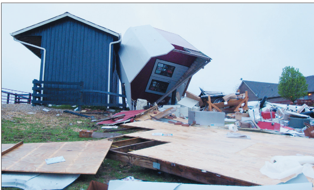
A 12x32 storage building was completely destroyed and another one, shown above on its side, located on the property of Dr. James and Marcia Chism, was heavily damaged in Sunday night's severe thunderstorm, which hit Rockcastle County. The building, which was destroyed, was storing framing equipment and crafts owned by Mrs. Chism. The Chism's property is located on Little Brushy Branch off Quail Road (618).
