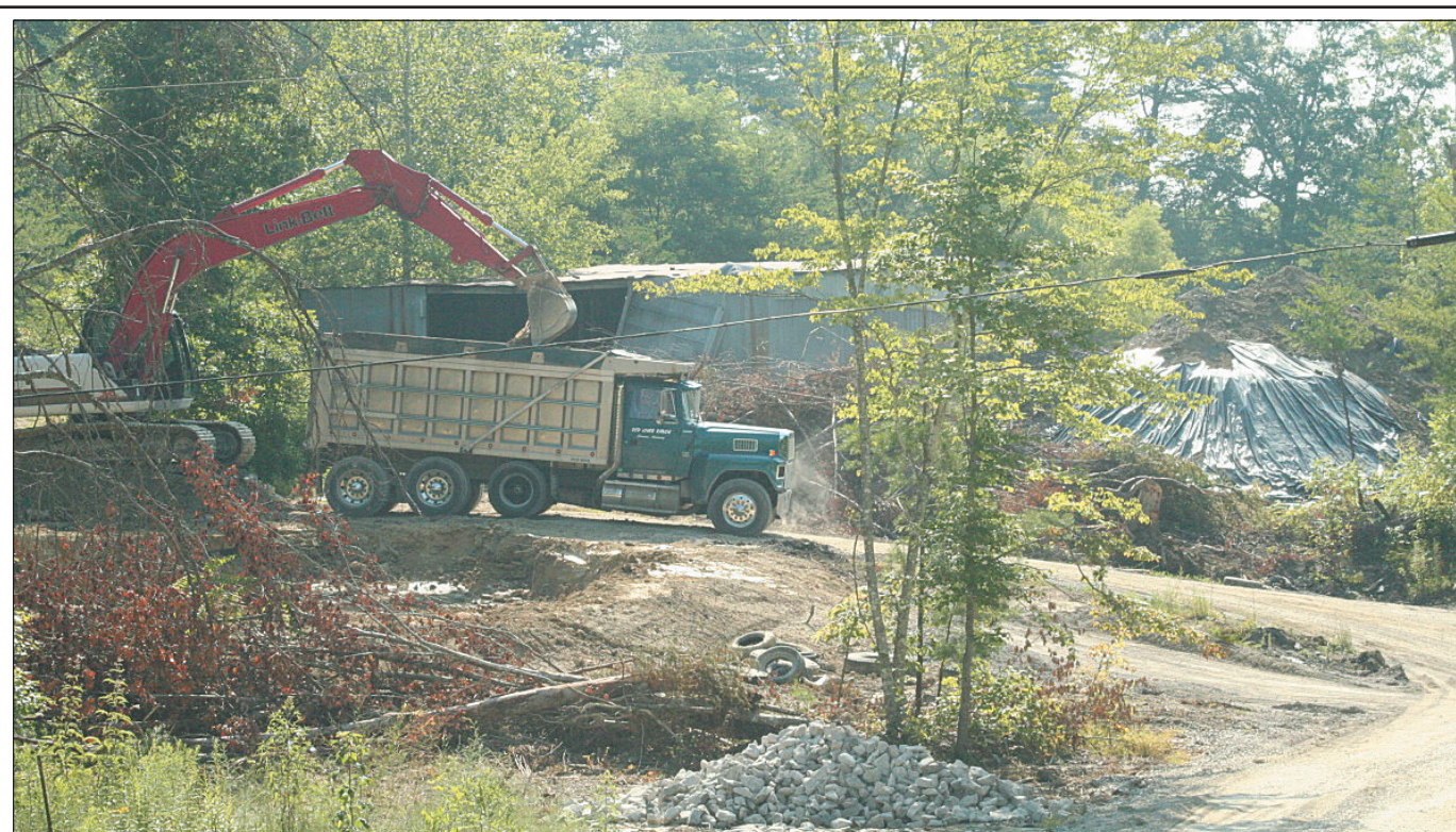
A Nicholasville company has been working for about a month to cleanup a 13 acre dumpsite on Buffalo Hollow Road. The cleanup was authorized by the federal EPA and is expected to take a couple more weeks.
