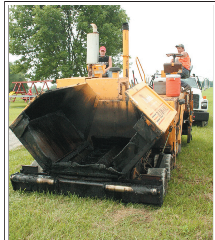
Greer Bros. employees waited for instructions before they began blacktopping a portion of Chestnut Grove Road on Tuesday morning.
