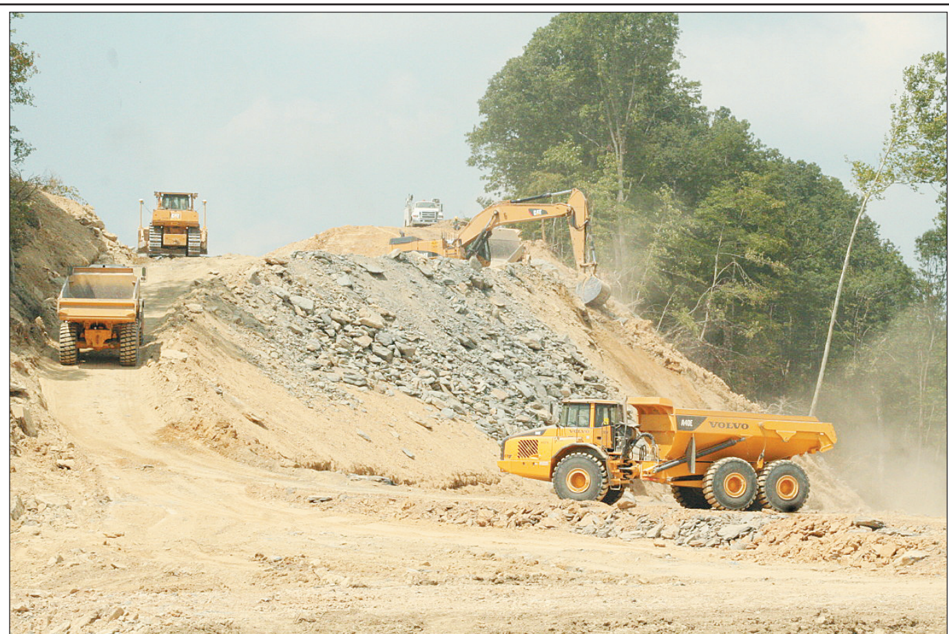
Construction on the new Hwy. 150, between Crab Orchard and Brodhead, began a few months ago. Employees with the Allen Company from Winchester were hard at work on Tuesday building the new roadway, about a mile west of Brodhead. Phase One of the project is expected to be completed in early 2010 and bids on Phase Two, between Brodhead and Hwy. 461 near Mt. Vernon, are set to be let in November. The total project for the 15 mile stretch of road from Crab Orchard to Hwy. 461 is $58.6 million. (Front page photos by: Richard Anderkin).
