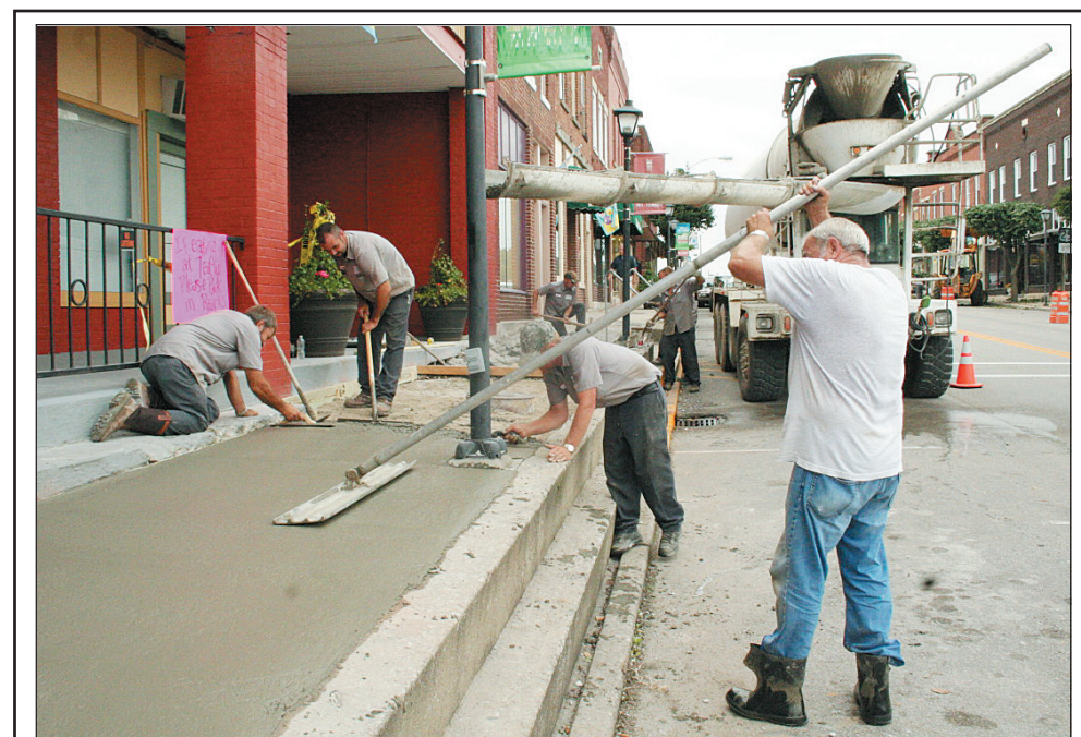
A portion of the West side of Main Street in Mt. Vernon was repaired last week by city employees and contractor Ray Lear. The sidewalk had been in poor condition for the past few years. Lear, shown at right, is being helped by City Superintendent Dennis McClure and city employees Brian Pittman and Ricky Miller. Mt. Vernon Mayor Clarice Kirby said the cost of repairs to the sidewalk totaled approximately $1,000 because of the work done by city employees.
