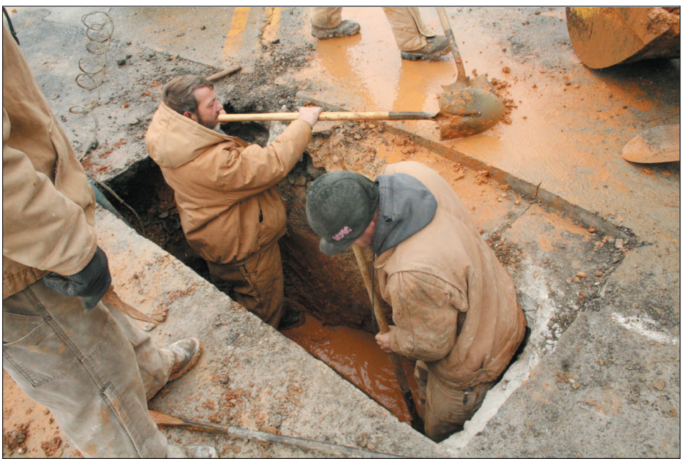
Mt. Vernon City Water Department employees braved the cold temperatures on Saturday morning to fix a main water line break, caused by the extremely cold temperatures the county has been experiencing. Above, city superintendent Dennis McClure, left and employee Brian Pittman work to get the broken line, which was on Main Street in front of McKinney's Tire. It took about six and half hours to fix the line but no customers were without water, although some residents did experience low water pressure.
