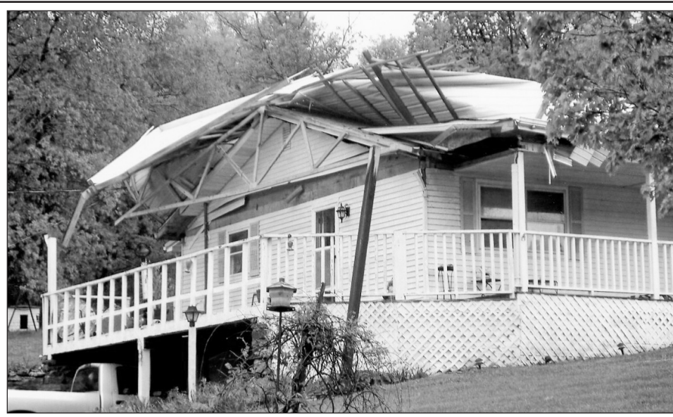
This home belonging to James and Roberta McClure on Blue Springs Road was severely damaged by a straight line wind on Sunday morning. County Judge-Executive Buzz Carloftis is asking residents of Rockcastle County who had damage to contact the emergency management services at 256-8436 and leave the following information: name, physical address, telephone number and brief description of damage to the property. Photos would also be very useful. State and federal agencies should begin assessments at the end of this week.
