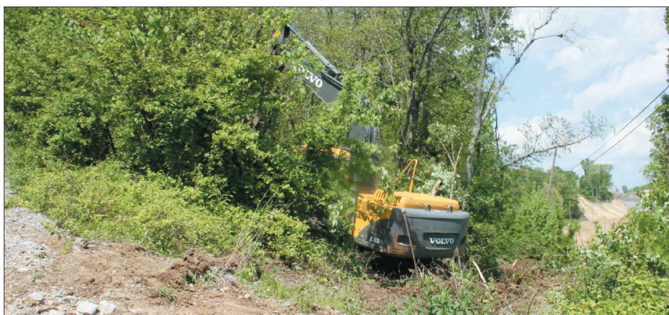
Employees of Western Rockcastle Water were busy Monday repairing water lines damaged in the weekend rain. Above, a completely new water line had to be replaced west of Brodhead after a hill slide destroyed the existing one. Employees had to clear trees and brush for the new water line. Over 500 customers were without water Monday morning but by Monday night all water had been restored.
