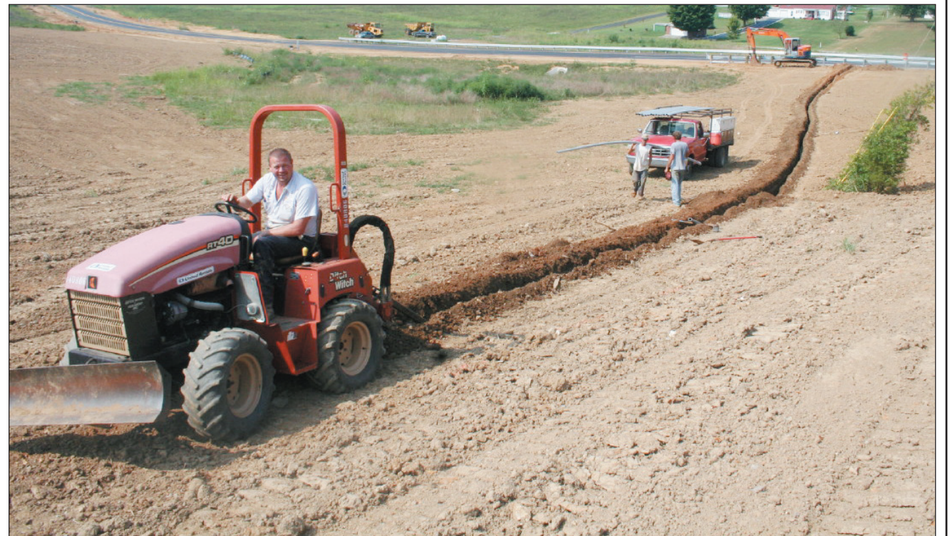
Much progress has been made in recent weeks with the completion of the Business Park South owned by the Rockcastle County Industrial Development Authority. The top picture shows the new turn lanes that were constructed by Goff Excavating. The bottom picture shows Jason Goff, of Goff Excavating, digging a ditch for the electrical conduit that will light the signage at the corner of Highway 150 and KY 2549. RCIDA recently hired Regina Crawford, a former staffer for Governor Ernie Fletcher and Senator Jim Bunning, to lead their efforts as Executive Director. She will take over effective September 1st (see related story).
