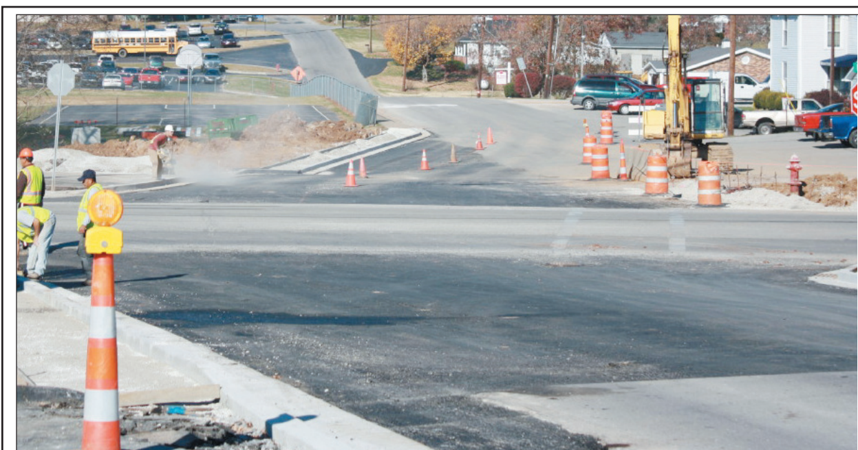
Work on the Newcomb Street - School Street project is beginning its final stages, with the rough coat of blacktop having been recently laid, and the final coat along with the striping set for next week. According to Mayor Gary Cromer, the state still has to put in two of the poles for the lights, and the hospital will soon begin erecting a new sign at the corner of Richmond Street and Newcomb Street.
