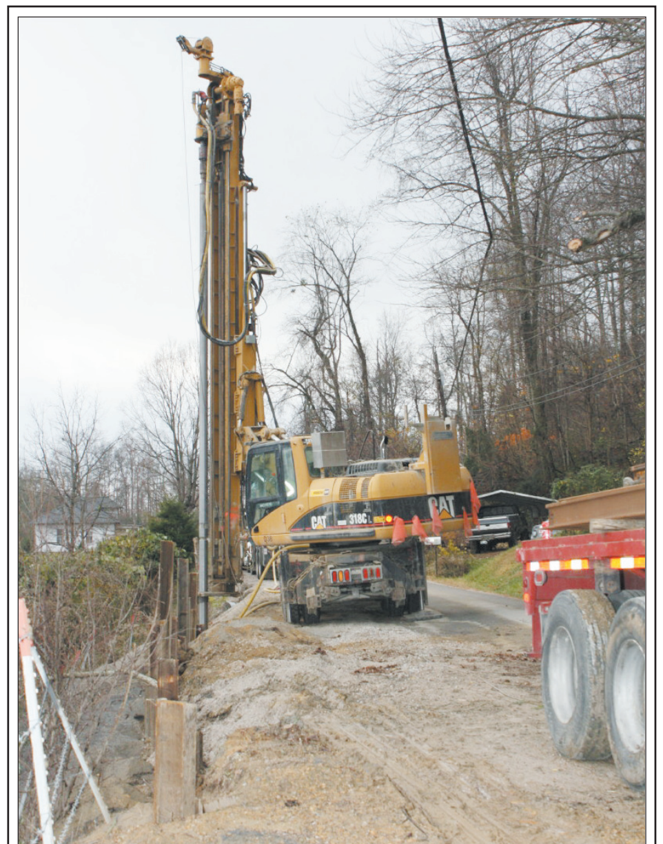
Workers were busy Wednesday morning repairing a major slip on Old Dixie Highway (Old U.S. 25). Crews had the road completely shut down. The slip is the second of four in the county that is being repaired primarily with FEMA funds. The first one repaired was on Mt. Zion Church Road. The final two to be repaired are on Buffalo Branch and Maret Cemetery roads.
