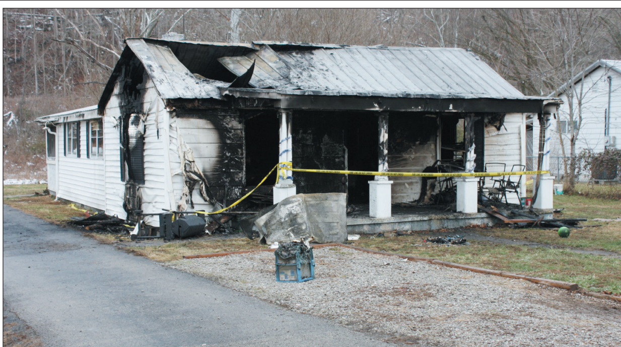
The Wildie home of Jon and Amanda Kerns was destroyed by fire early Sunday morning, as fire crews from Mt. Vernon, Brodhead and Brindle Ridge all responded to the fire. Kerns, who is a volunteer fireman with both the Brodhead and Mt. Vernon fire departments was the first fireman on the scene and began attacking the fire before the crews arrived. The Kerns's have one son, Austin, who is three.
