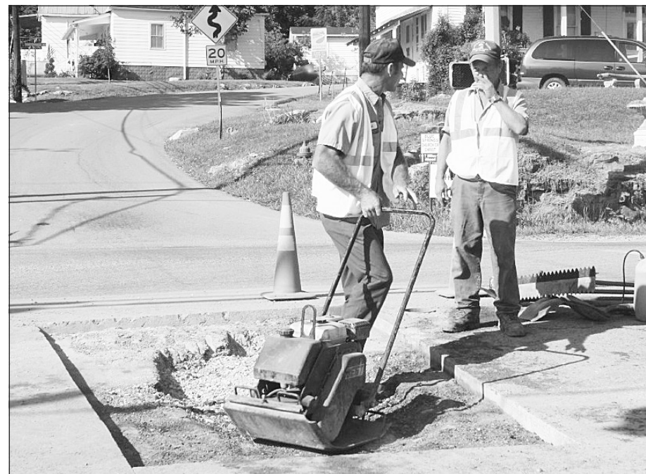
Mt. Vernon city employees Lloyd Prewitt and Dale Cotton, as well as others, spent most of morning repairing a water leak of U.S. 25 and Hwy. 150 in Mt. Vernon. Traffic going south on U.S. 25 was redirected down Main Street or West Main while repairs were ongoing.
