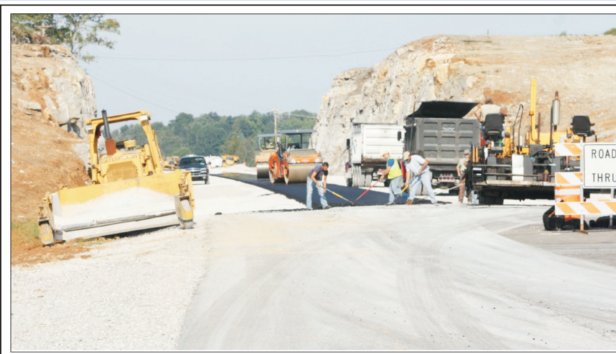
Workers were busy Wednesday laying blacktop on the last part of the new Hwy. 150 between Mt. Vernon and Brodhead. According to Transportation Cabinet officials, the road is scheduled to be opened sometime in October.
