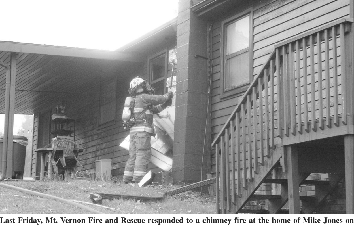
Last Friday, Mt. Vernon Fire and Rescue responded to a chimney fire at the home of Mike Jones on Hewitt Lane in Mt. Vernon. The home sustained quite a bit of smoke damage. Mt. Vernon Fire Department was assisted at the scene by the Brodhead Fire Department.
