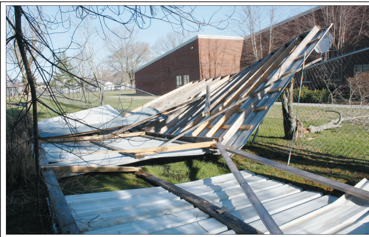
A storage building collapsed onto a fence at the Brodhead Elementary School on Albright Street in Brodhead during the storm Friday night. Other than the collapsed building in Brodhead, only minor home and vehicle damage was reported in the county.
