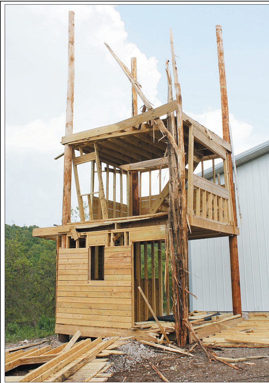
A severe storm system moved across the county Thursday afternoon destroying the training tower at the Mt. Vernon Fire Department and causing a water line break in front of the fire station on old U.S. 25. Mt. Vernon Fire Chief David Bales said the tower had only been completed for a few months and will cost approximately $9,000 to rebuild.
