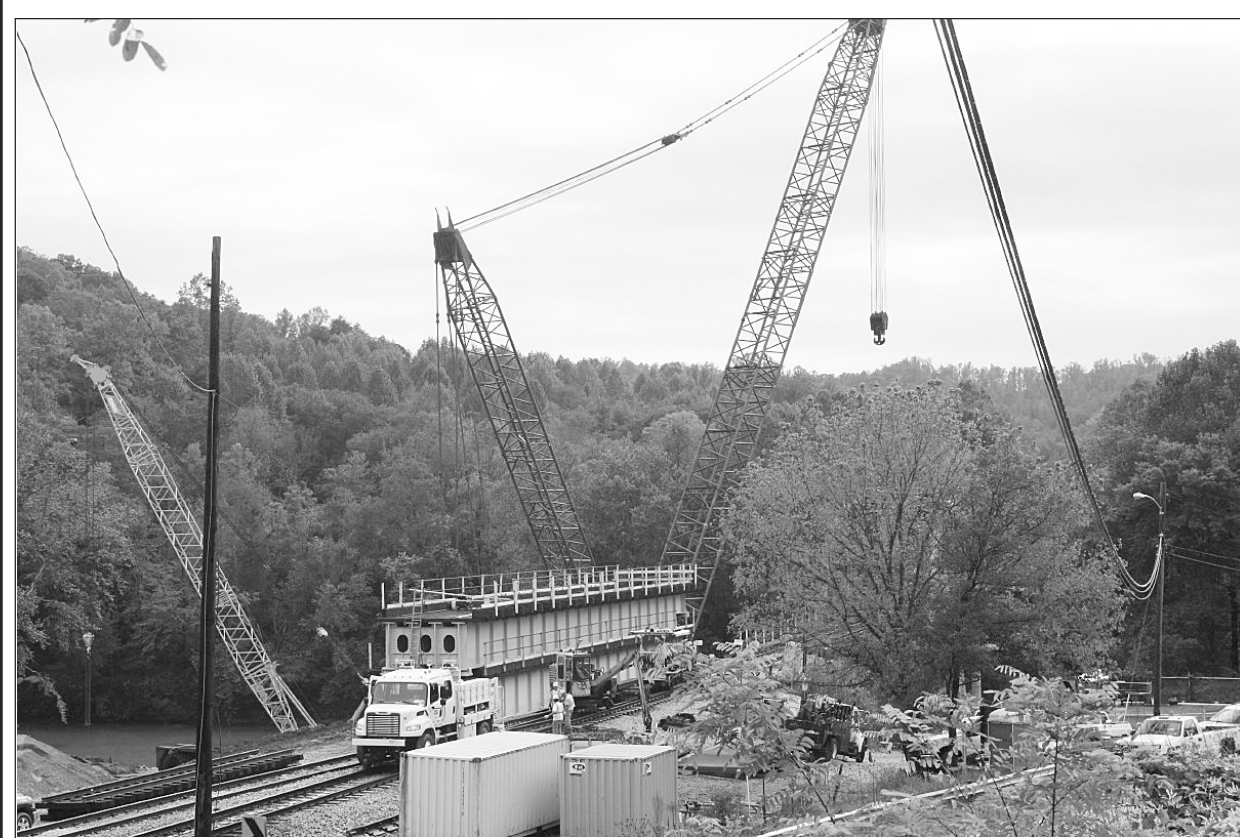
The 100,000 ton crane that is being used to replace the 106-year-old railroad bridge in Livingston, now has its boom attached. Production was halted last Tuesday because of heavy rains. During the rain, 43 support pads for the crane floated down the Rockcastle River. 28 were later recovered between Livingston and Skaggs Creek, 15 are still reported missing. The pads are estimated at $1,100 each and all 43 had to be replaced.
