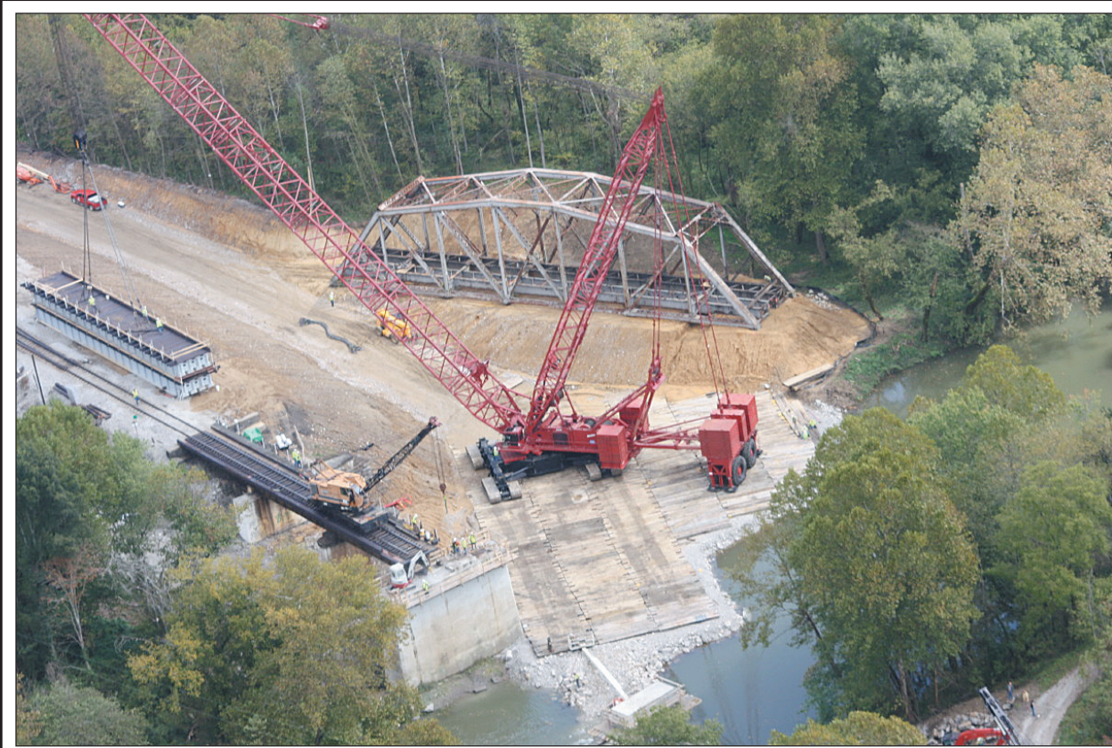
The process of replacing the 106-year-old truss railroad bridge over the Rockcastle River in Livingston is now complete. CSX crews completed the project this past weekend and the first train used the new ballast deck railroad bridge early Sunday morning. The aerial photo above was taken Saturday afternoon before CSX crews positioned the new Ballast Deck bridge. The bridge was replaced due to its age and for safety reasons.
