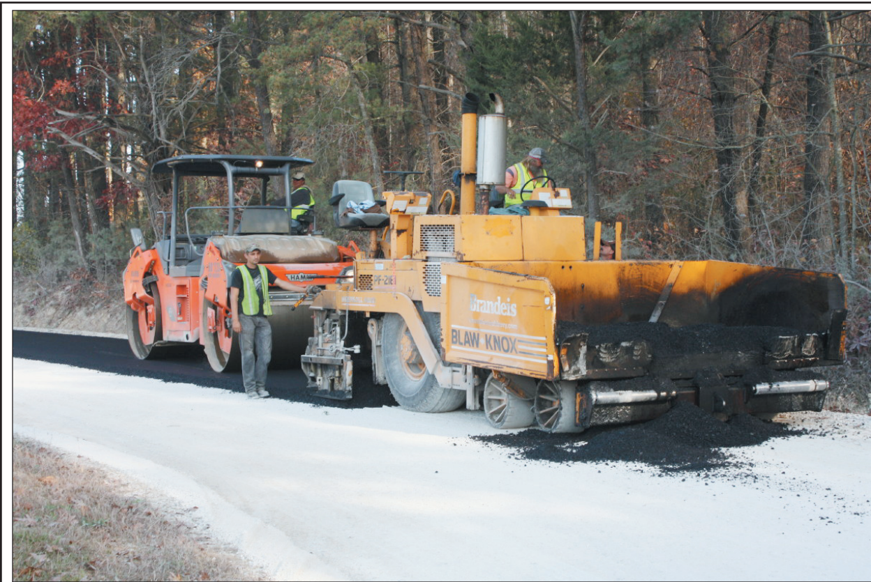
Greer Bros. Construction began the three-mile resurfacing project on Lambert Road in northern Rockcastle County Tuesday. County Judge/Executive Buzz Carrloftis estimated the cost of the project, which included widening the road, installing culverts, rock hauled and the resurfacing, at about $750,000 total. The resurfacing is made up of a two inch asphalt base and one inch of blacktop.
