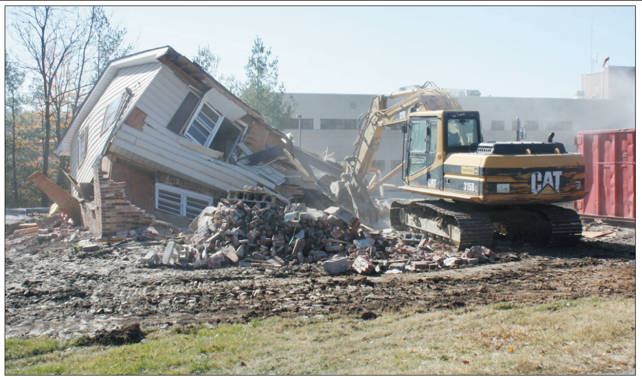
Goff Excavating began demolition Tuesday at the site for Rockcastle Regional Hospital's new medical office building on High Street in Mt. Vernon. After Goff Excavation completes the work, Rockcastle Regional Hospital will begin construction of the new building. Doctors David Bullock, Kevin Rowe, Karen Saylor and a host of other nurse practitioners and physician assistants will provide care in the building when it opens in December 2013.
