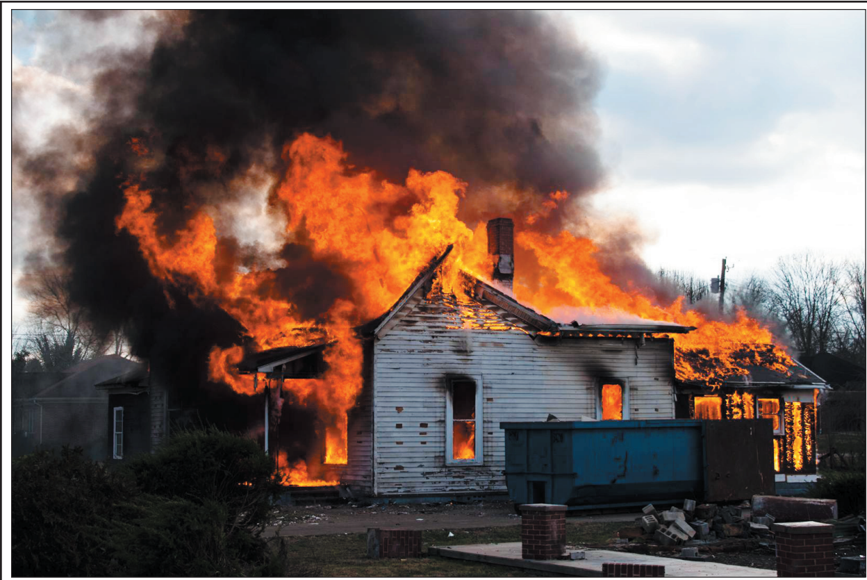
Brodhead Fire Department and Mt. Vernon Fire and Rescue responded to a house fire last Friday on Maple Street in Brodhead. Authorities say the abandoned house was owned by Brodhead Baptist Church, who was in the process of demolishing the house. Officials believe workers were burning debris next to the house when it caught fire. No one was injured in the fire.
