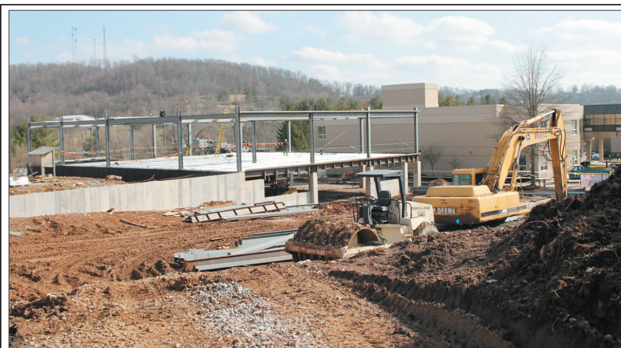
Everything is going as planned for the construction of the new Rockcastle Family Wellness building at Rockcastle Regional Hospital. The new $3.2 million building will be located on High Street behind the Medical Arts building and will serve as offices for Doctors David Bullock, Kevin Rowe, Karen Saylor and a host of other nurse practitioners and physicians assistants. The building is scheduled to be completed in December of this year.
