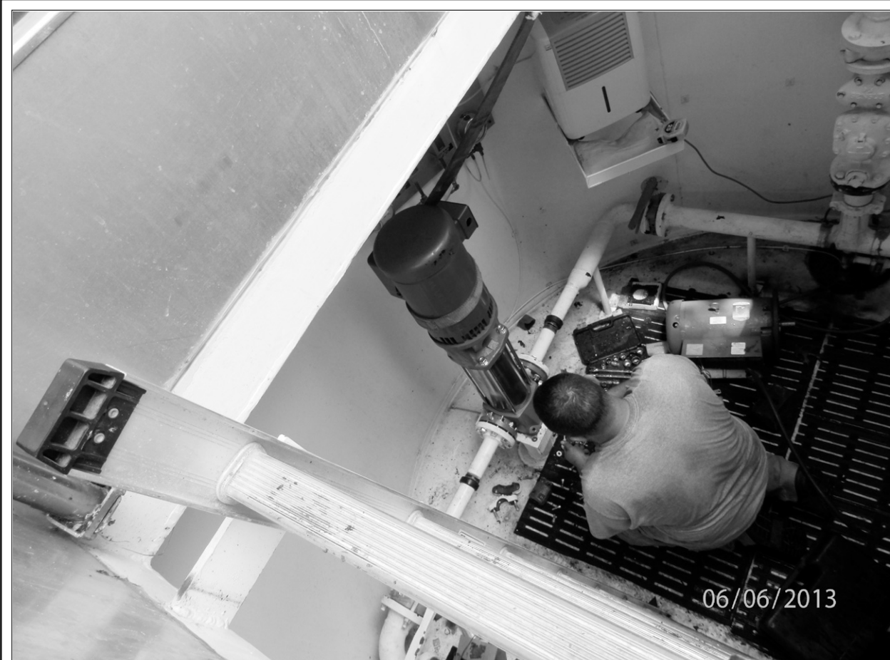
Eastern Rockcastle Water Association recently finished installing a new pump at their Sandhill pump station near Livingston. The motor quit on the old pump causing a new pump to have to be installed. The newly installed pump should prevent any interruption in service for the customer area, except during a power outage.
