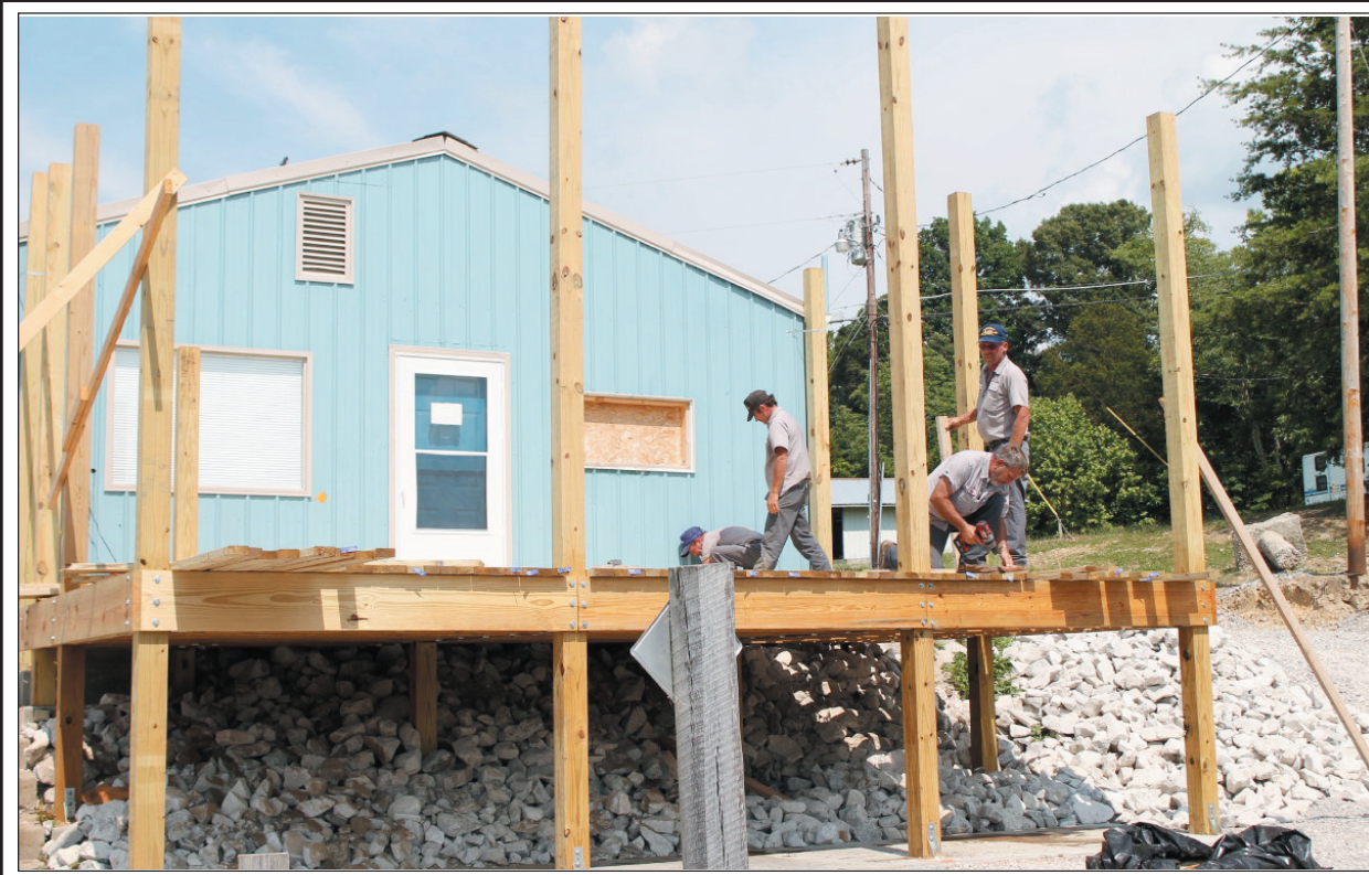
Mt. Vernon city workers are finishing up the new deck at the Lake Linville boat dock. The deck will include a dining area with an awning. The deck is scheduled to be completed before the Grand Re-opening of the boat dock next Wednesday.
