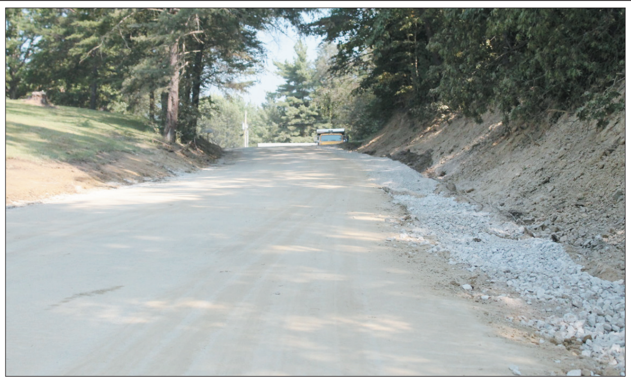
Rockcastle County road and maintenance crews have begun construction on the widening of Flat Gap Road in northern Rockcastle. County Judge Executive Buzz Carloftis said they are widening the road two feet on both sides of the road where it is most needed. Carloftis said the project should be completely finished by the summer of 2014.
