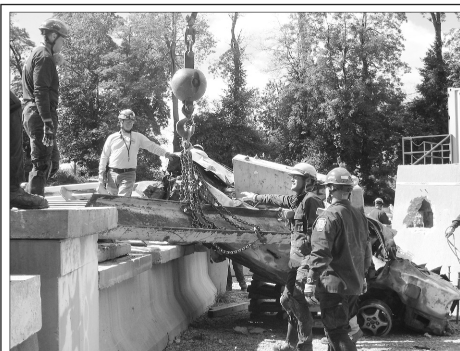
Capt. Rick Branham works with a crane and rigging to move a 1700 lbs. steel beam off a car in the final scenario.
