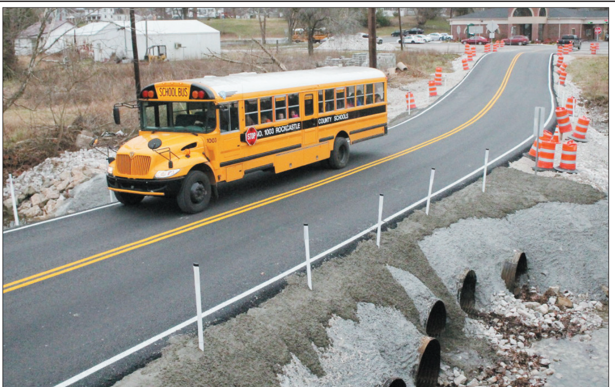
The temporary bridge in Brodhead was recently blacktopped. The bridge was built to eliminate the lengthy detours for motorists that was caused by the closing of the Dix River Bridge. The temporary bridge will be in use until the Dix River Bridge is reconstructed and reopened for use. Bids for the reconstruction will be let in January and the project is scheduled for completion in the spring of 2014.
