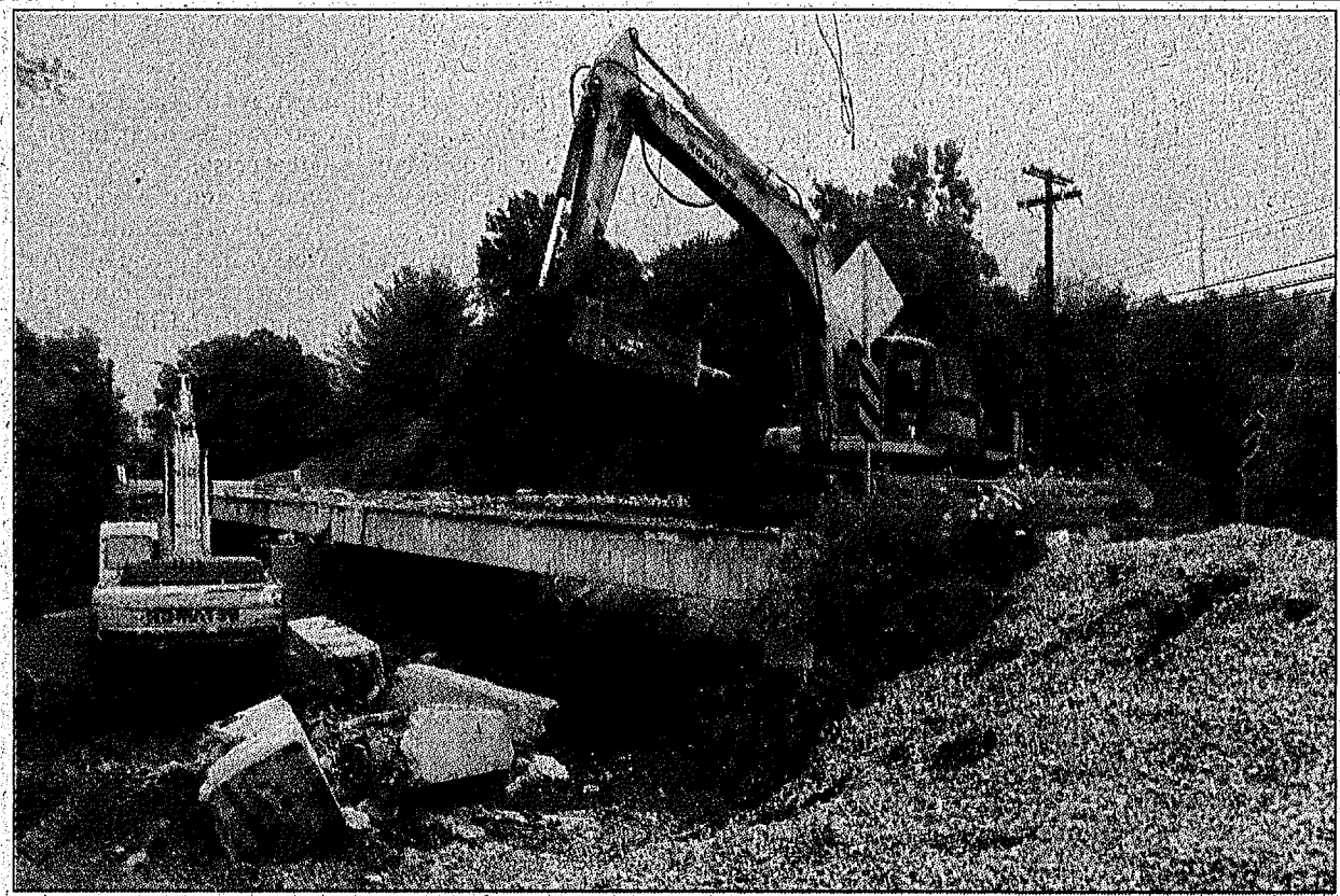
Reconstruction was started last Friday on the Dix River Bridge that was condemned in Brodhead. Contractors hope to have the bridge reconstructed by the beginning of August. The bid for the reconstruction project was awarded to K and K Construction of London for $540,750 and the emergency funding to reconstruct the bridge was provided by the KYTC Rural and Secondary Roads Program.
