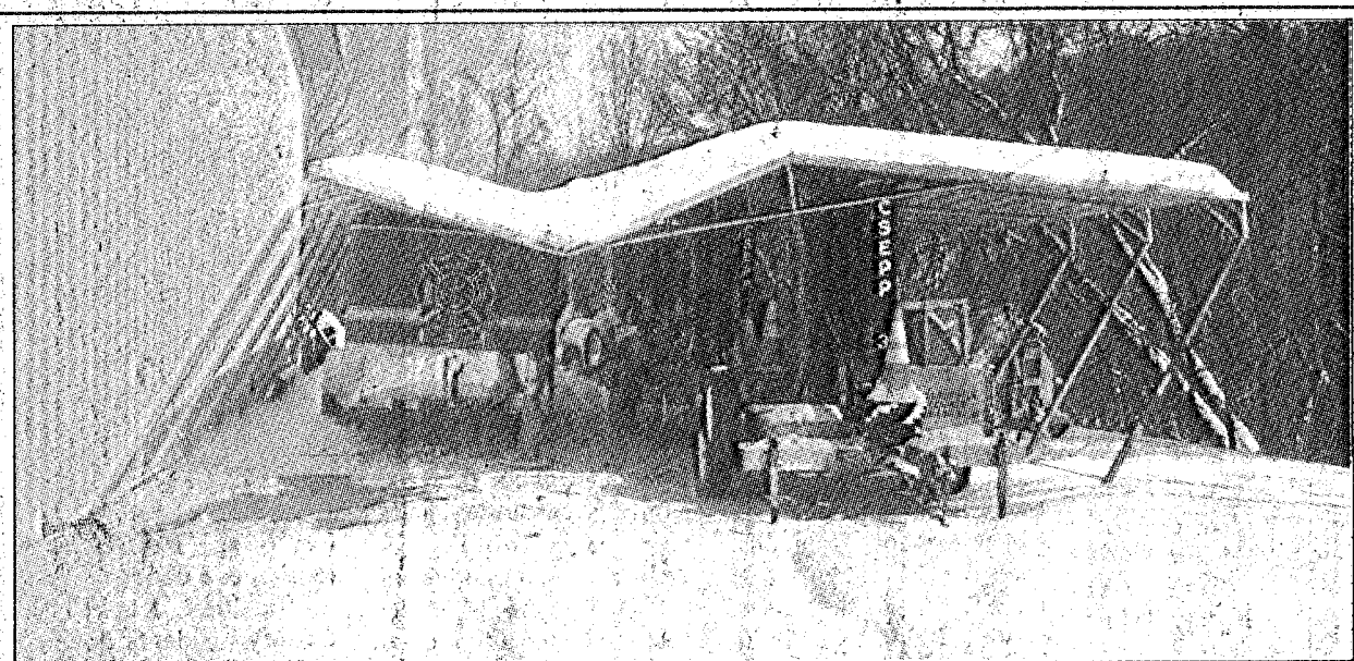
The Mt. Vernon Fire Department had a metal carport collapse last Wednesday afternoon due to the heavy weight of the snow from Winter Storm Octavia. Mt. Vernon Fire Chief David Bales said the collapsed carport damaged the top of a rescue trailer and also damaged some of the solar panels on the road sign boards.
